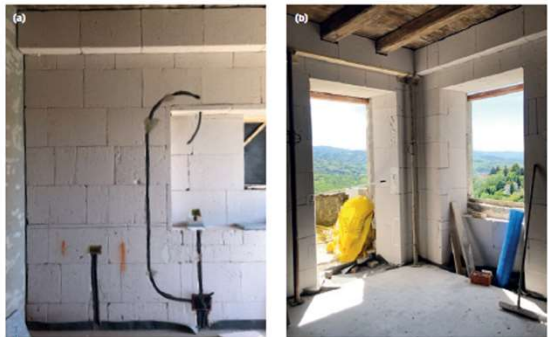
Fig. 5: (a) Electrical system sheaths (b) shoulder pads of the windows
